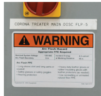
Arc Flash Panel Labels
